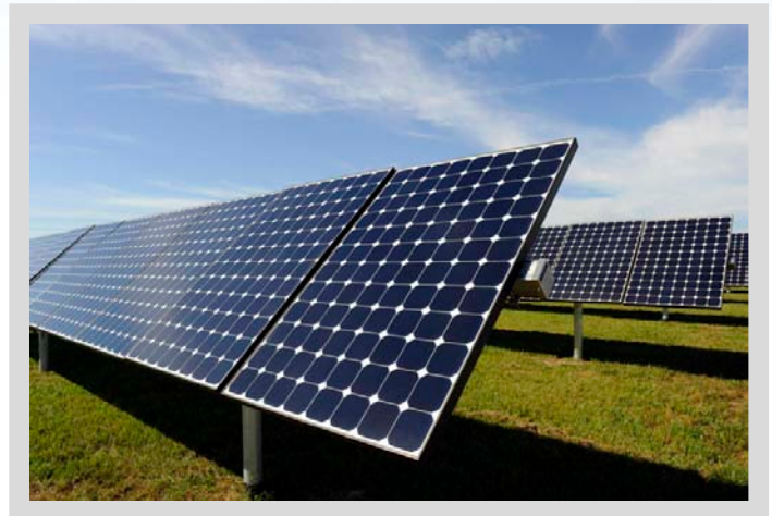
The 25 MW photovoltaic DeSoto Next Generation Solar Energy Center in DeSoto County, Fla., was completed in October 2009.
