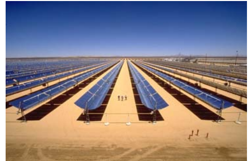
A parabolic trough plant in California's Mojave Desert.
