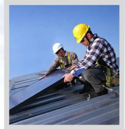
Solar installation workers mount PV panels on a private home. These panels generate clean, pollution-free electricity and can reduce or eliminate monthly electricity bills. In 2008, over 16,000 residential systems were installed, with an average size of just under 5 kilowatts (kW). (Photo – NREL)
