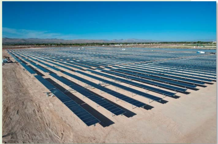
View of 14 MW PV system at Naval Weapons Station China Lake. (Photo: SunPower Corp.)
