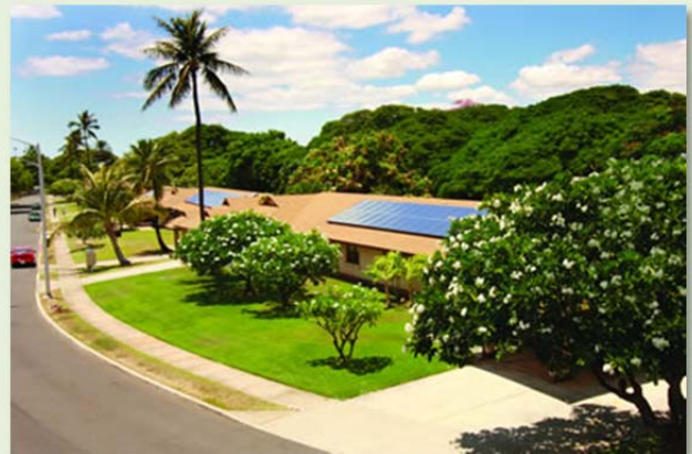
One of the hundreds of PV systems installed at homes at Hickam Air Force Base. (Photo: SolarCity)
