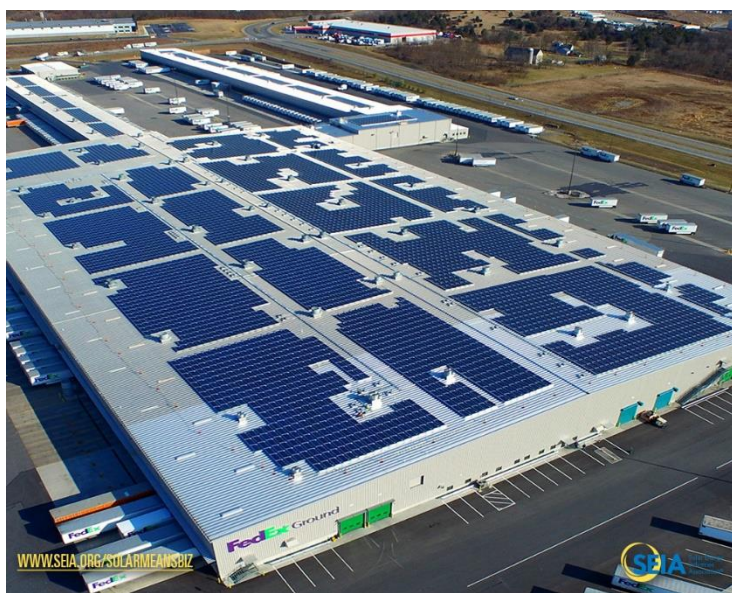
The 2.7 MW solar array at FedEx's facility in Hagerstown, MD consists of nearly 9,000 individual modules and offsets 37% of their electricity demand. Photo credit: FedEx
