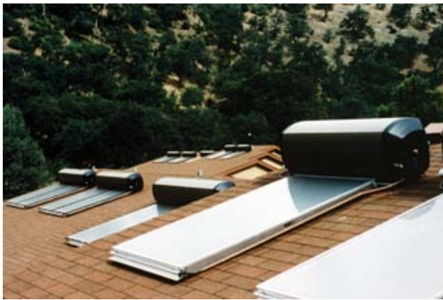
Solar water heaters on employee housing in Yosemite national park Courtesy of DOE/NREL, Credit: Jim Schwerm
