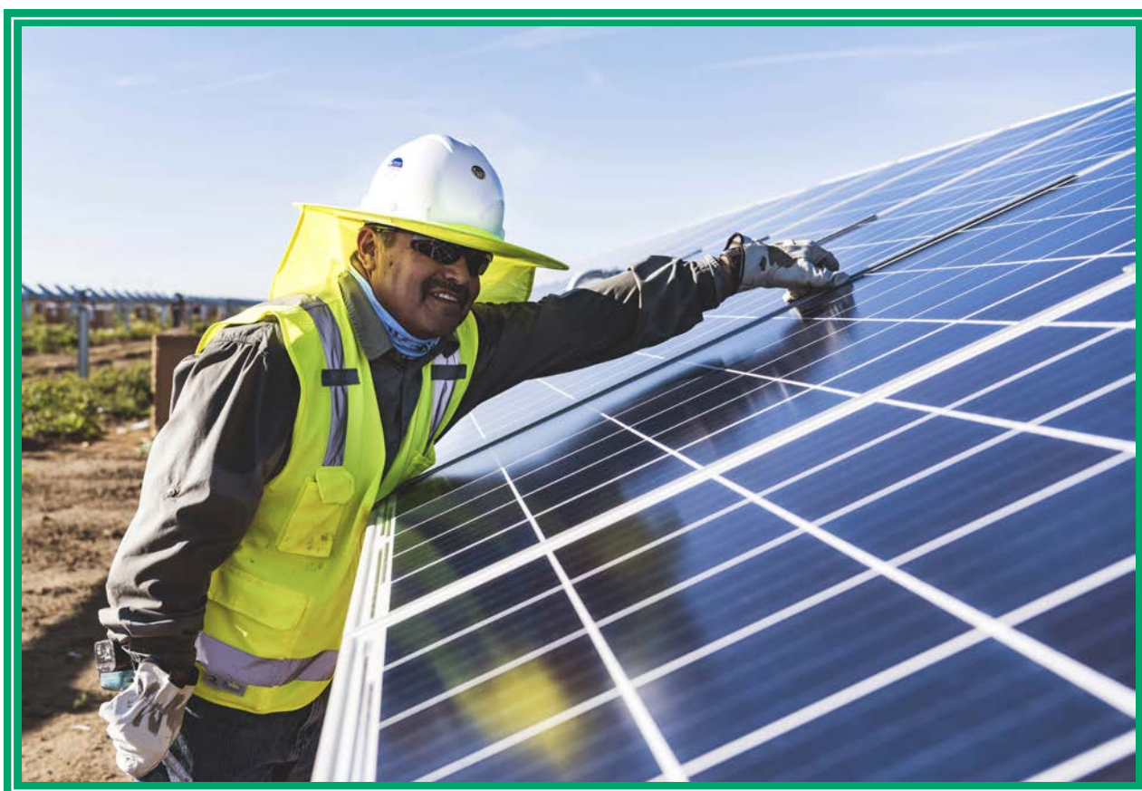
Photo courtesy of Swinerton Renewable Energy
