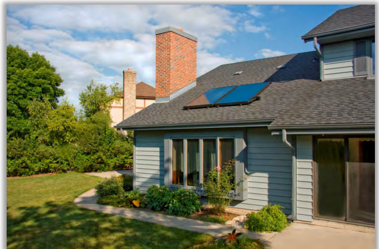
Solar water heating system on home. (Caleffi Solar)
