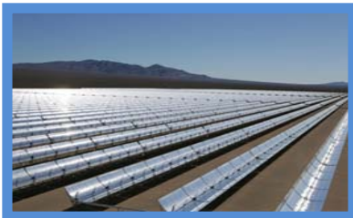
Project Name: Nevada Solar One Developer: Acciona Electricity Purchaser: NV Energy Location: Boulder City, Nev. Technology: Trough Capacity: 64 MW Source: Acciona North America
