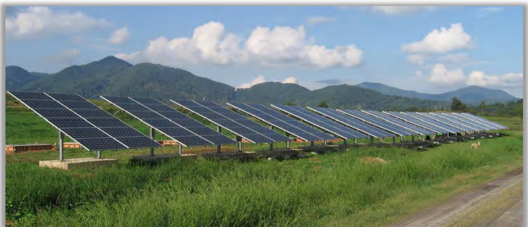
A 555-kW PV system on landfill in Canton, North Carolina. (Joanna Malcolm, FLS Energy; Suniva)
