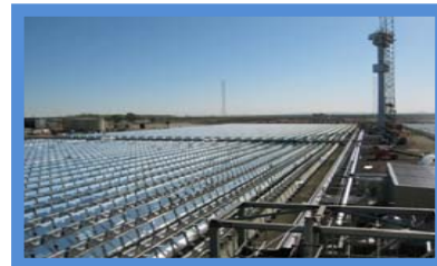
Project Name: Sierra SunTower Developer: eSolar Electricity Purchaser: Southern California Edison Location: Antelope Valley, Calif. Technology: Tower Capacity: 5 MW Source: eSolar
